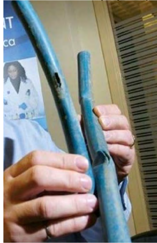
Deteriorated Pieces of Polybutylene Pipe
