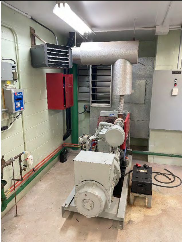
Sewage Pump Station Back-up Generator
