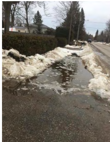
Flooded Ditch and Culvert
