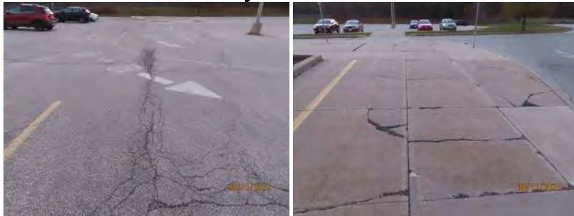
Damaged asphalt and concrete – Sutton Multi Use
