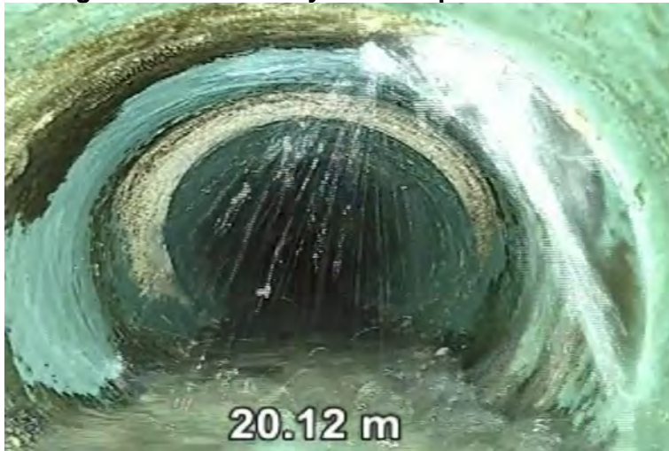
Damaged Plastic Sanitary Sewer Pipe with Inflow Occurring
