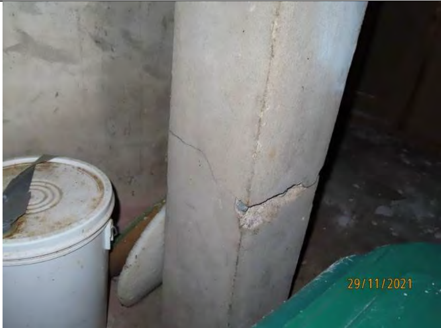
Belhaven Hall damaged column
